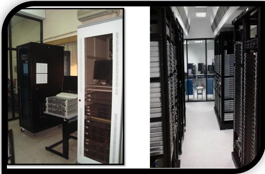
High Performance Computation Facility at HRI
