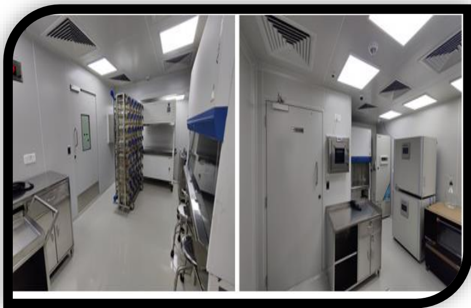
Biosafety Lab (Level III) at RMC-BARC
