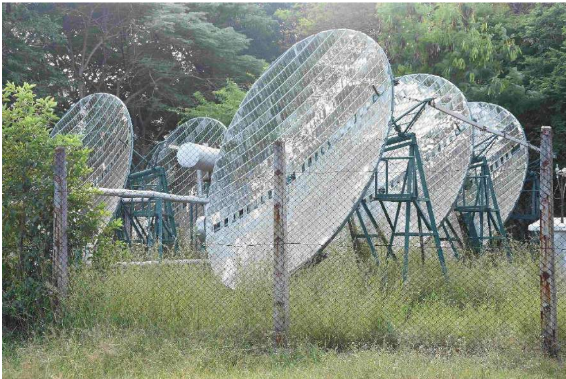
Solar-Thermal Power Facility for Cafeteria at IGCAR, Kalpakkam
