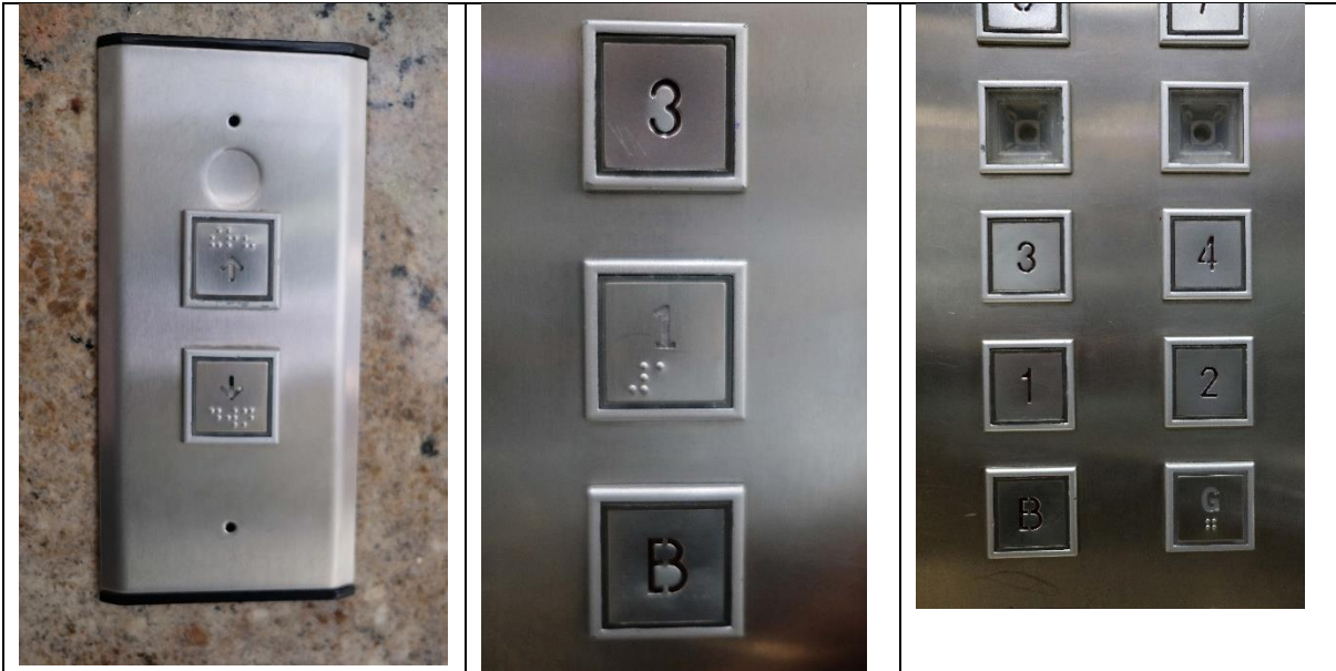
Disabled Friendly Lift Facility at Tata Memorial Centre, Mumbai
